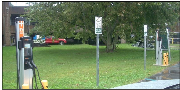
Gateway Charging Station
